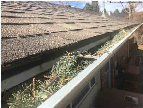
Winter winds can add a surprising amount of debris to the gutters.
